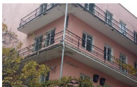
One of the schools in Tbilisi damaged by earthquake
